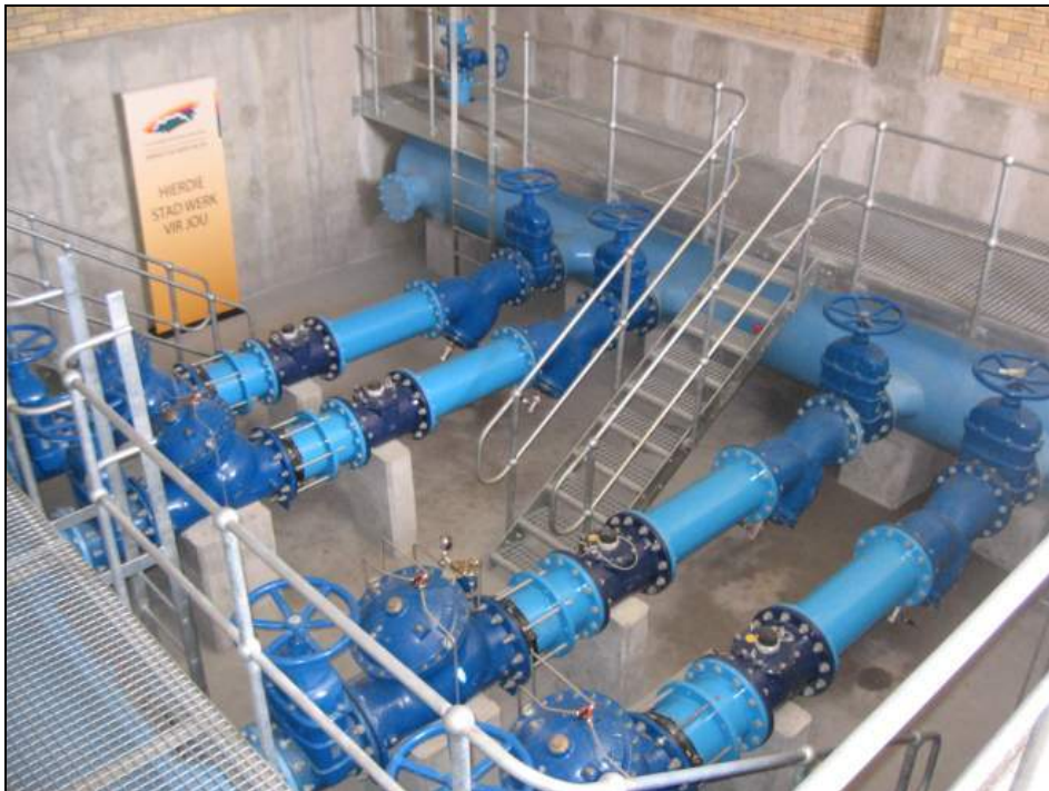
Figure 2: Installed pipework in recently completed Mitchells Plain Pressure Management Chamber on the 1220mm diameter pipe.
