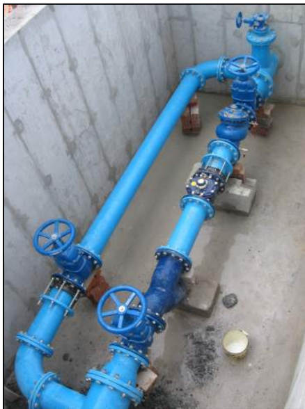
Figure 4: Installed pipework in recently completed Mitchells Plain Pressure Management Chamber on the 300mm diameter pipe.
